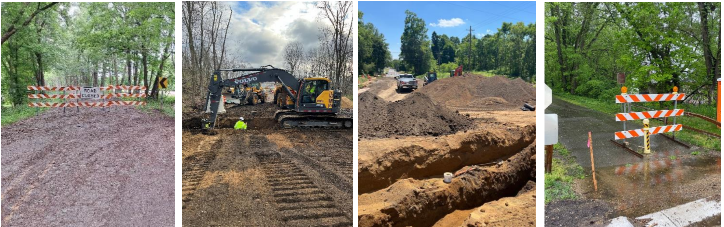
Pictured: This week's work on Squires Drive and Drake Road, and 19 th Street in Cooper Township. Please respect the barricades and follow posted detour routes.
